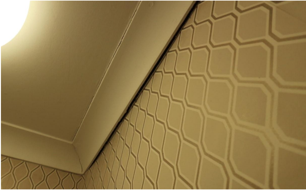
Damage to the Bathroom
